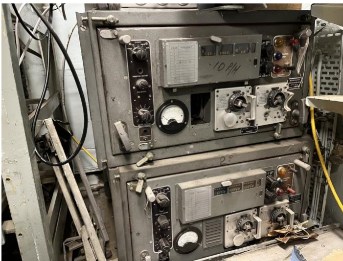
Some AM Tx's to restore....
